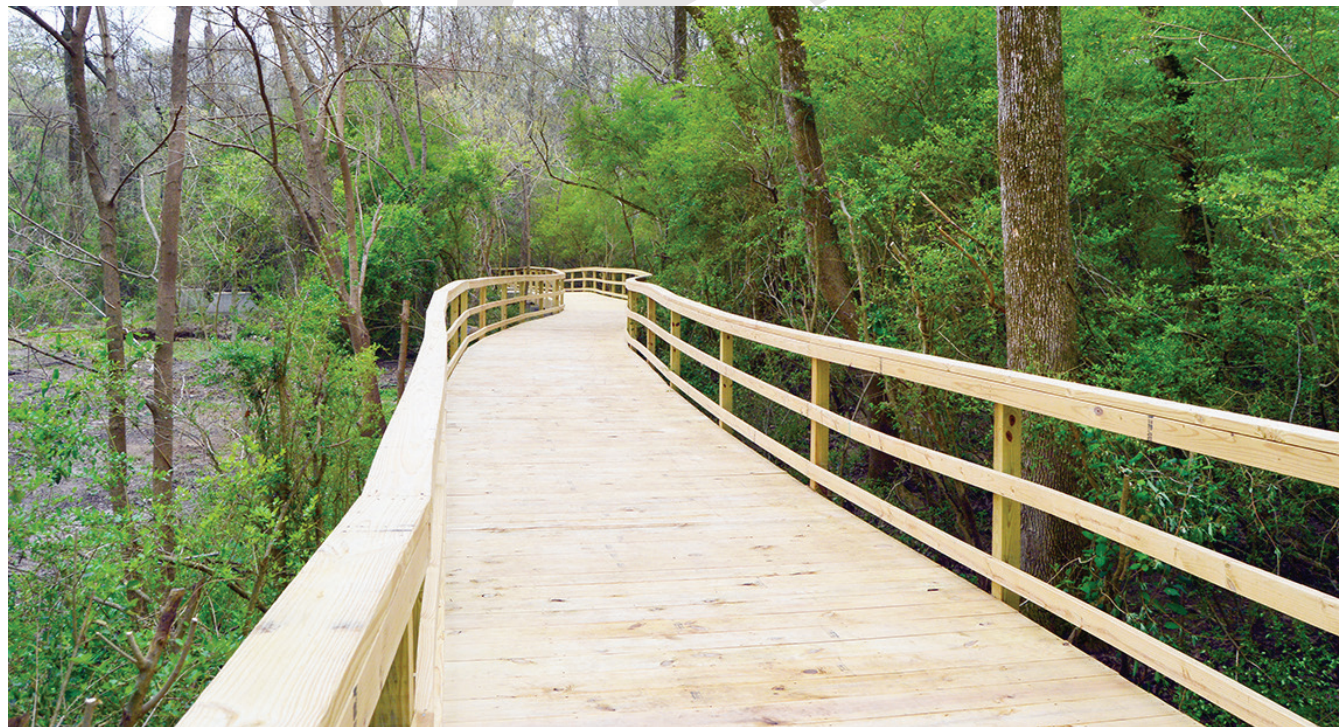
ABOVE A new boardwalk installed as part of the trail network around Rosel Fann Recreation Center in 2016.
